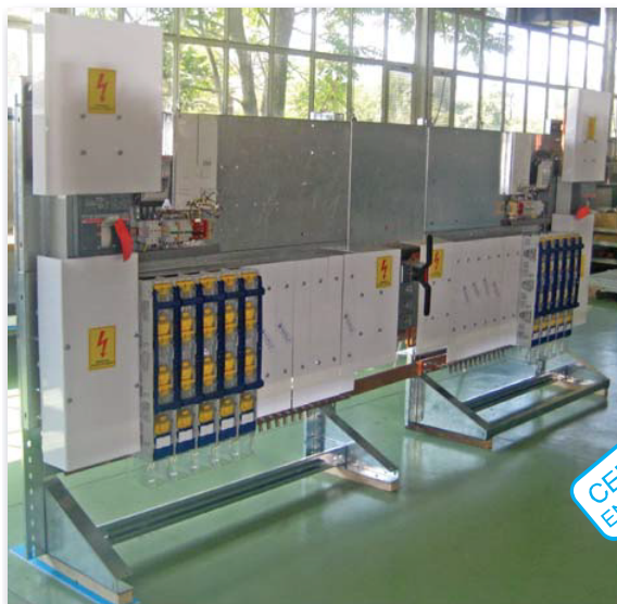
Low voltage switch boards 2x1000kVA with coupling 1600A
