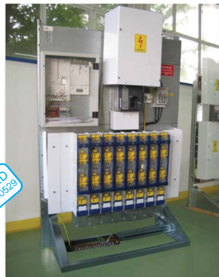
Low voltage switch boards 1000kVA
