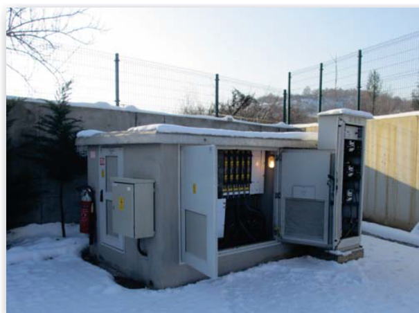
Transformer substation TEP800-1 20(10)/0.4kV, 630kVA, Skopje
