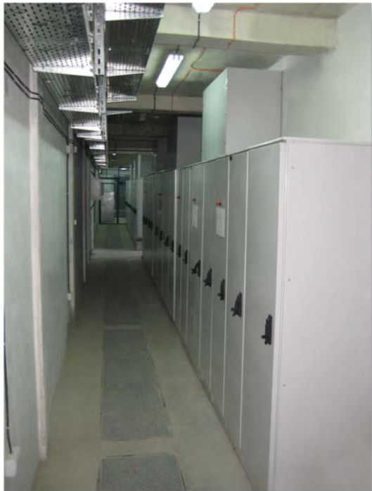
0.4kV Main distribution board City Mall Skopje
