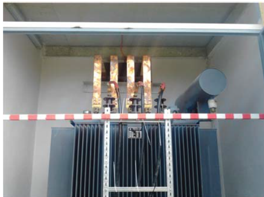
Transformer part - 1600 kVA, 20kV
