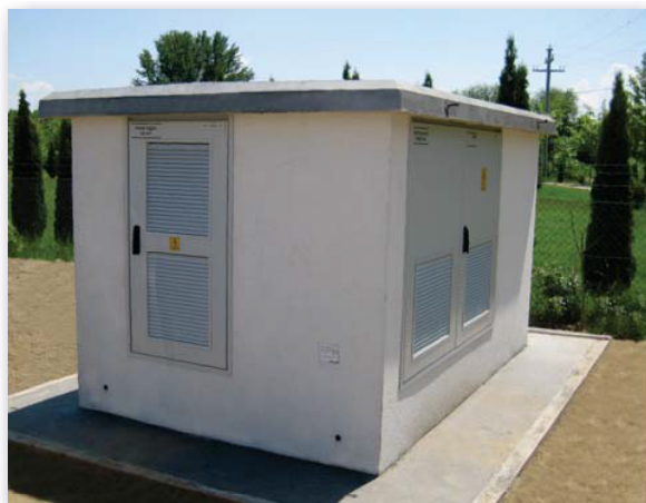
Transformer substation TEP800-1 20(10)/0.4kV, 630kVA, Kumanovo
