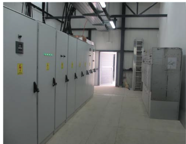
Transformer substation 1000 kVA, 20kV Pilot training center in Petrovec
