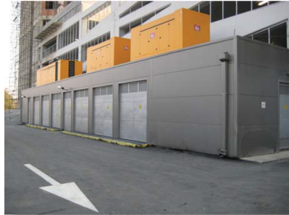
Substation 6x1600kVA City Mall, Skopje
